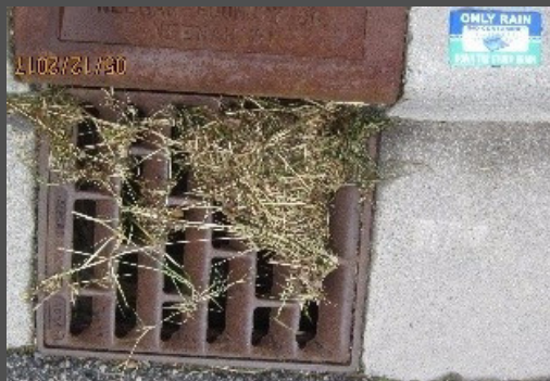
Grass clippings stuck in a storm drain.
